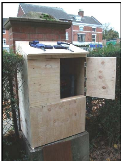
New electric housing unit for the library corner fountain
